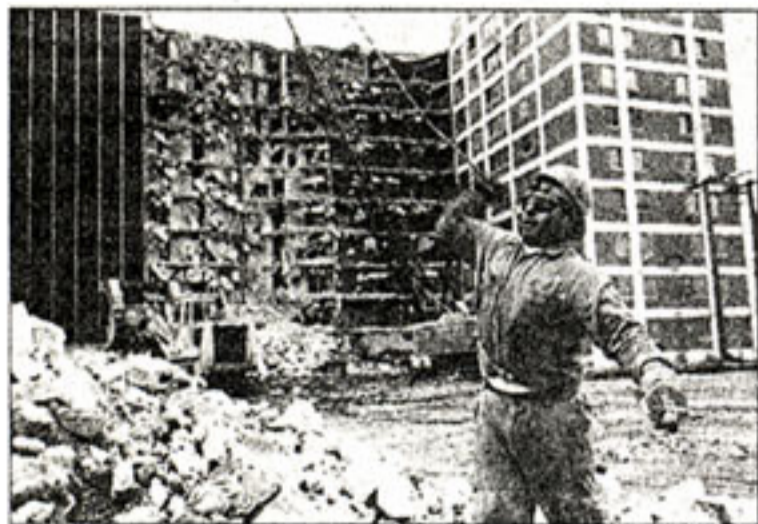
Worker Greg Hernandez separates the different types of rubble after the demolition of Cabrini-Green buildings in the 1100 block of North Cleveland Avenue.
